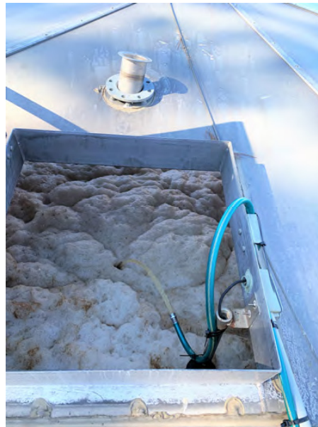
Dosing 260,000 gal tanks
