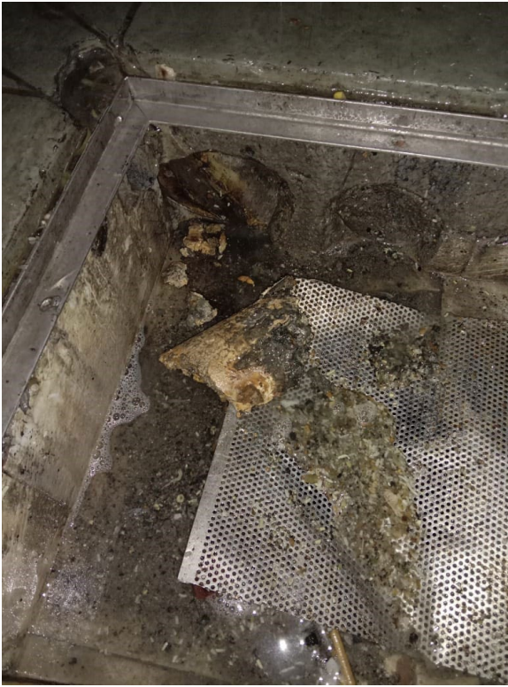
Flow of accumulated FOG through kitchen pipe
