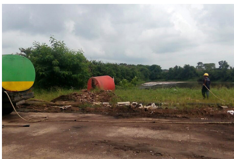
Water tank connected to a hose for dosing
