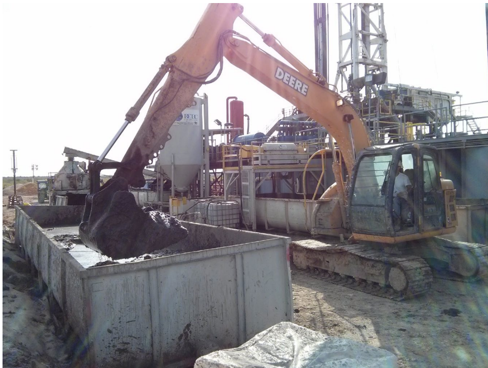
Treatment of dryer cuttings
